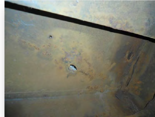
Corrosion Hole/Crack in Articulated Structure
