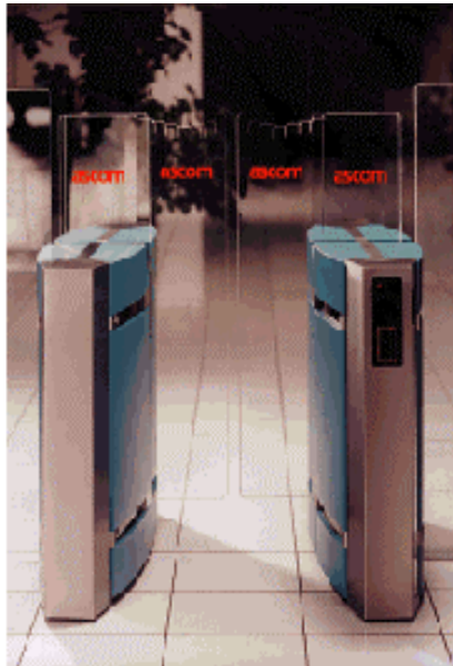
Access control gates
