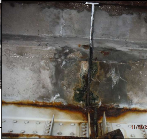
Looking up @ failed expansion Joint
